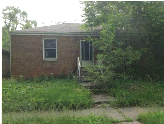
Does not meet the property maintenance codes
